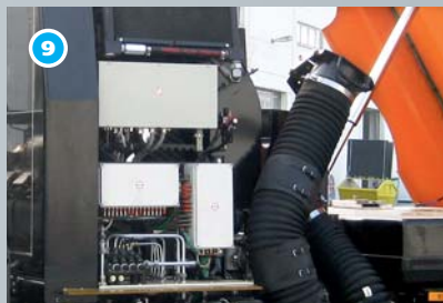
The efficiently arranged control centre
